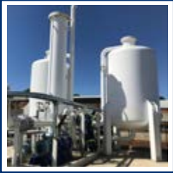
Vapour Recovery Unit
